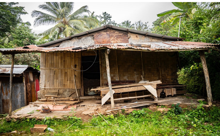
One of the houses in Balibar village that was damaged by the floods on the way between Katarina and Maria's house. Photo by Sarah Al Jameel/ IOM Timor-Leste 2024.
